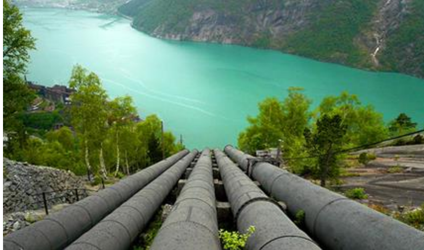
Figure 1 Picture of penstock pipes.
