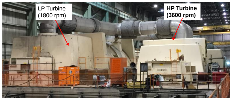
Figure 3: cross-compound steam turbine generator
