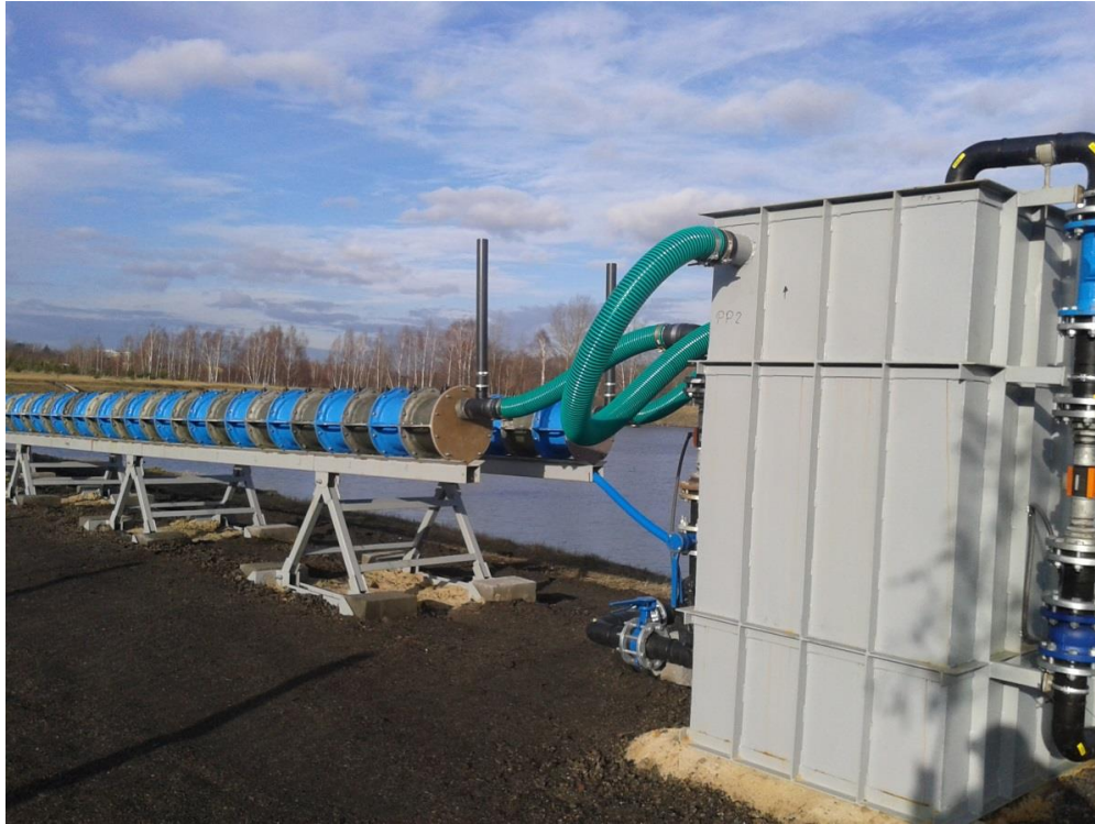
Fig.1. Surface installation for radium removal from brines
