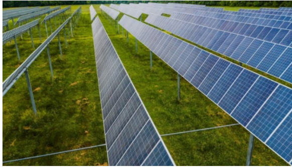
Fig. 14: Example of an elevated solar structure.
