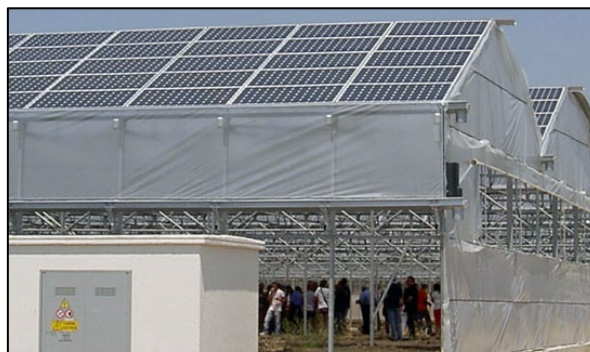
Fig. 15: Example of a photovoltaic solar installation on a greenhouse roof.
