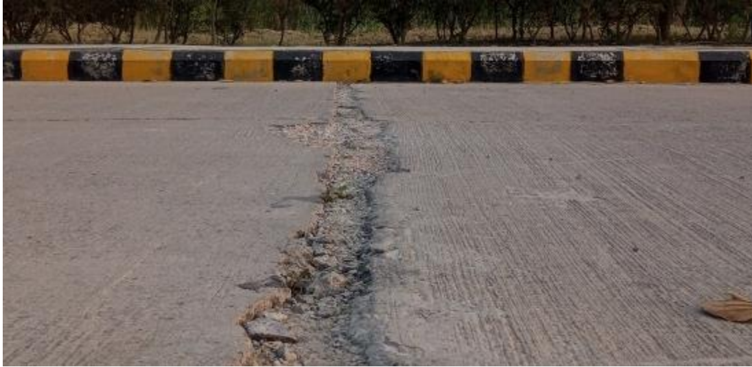
Fig. 6 Actual image of road condition.
